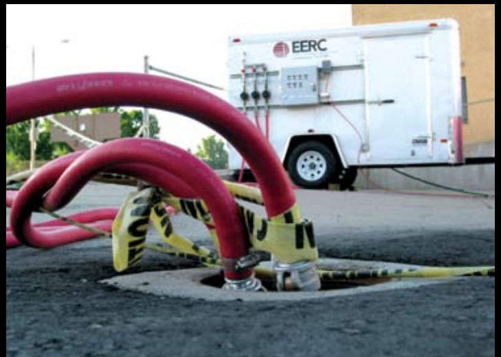
Mobile multiphase contaminant recovery and injection systems applied for controlled injection of O 2 and nutrient-enriched water for in situ contaminant treatment in Bismarck, North Dakota.
