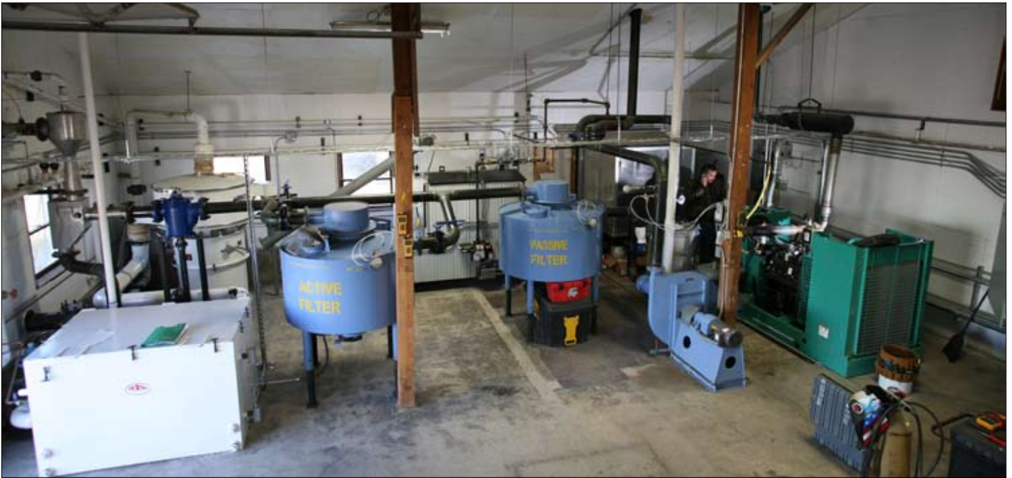
The inner workings of the biomass gasification system at G F Truss.
