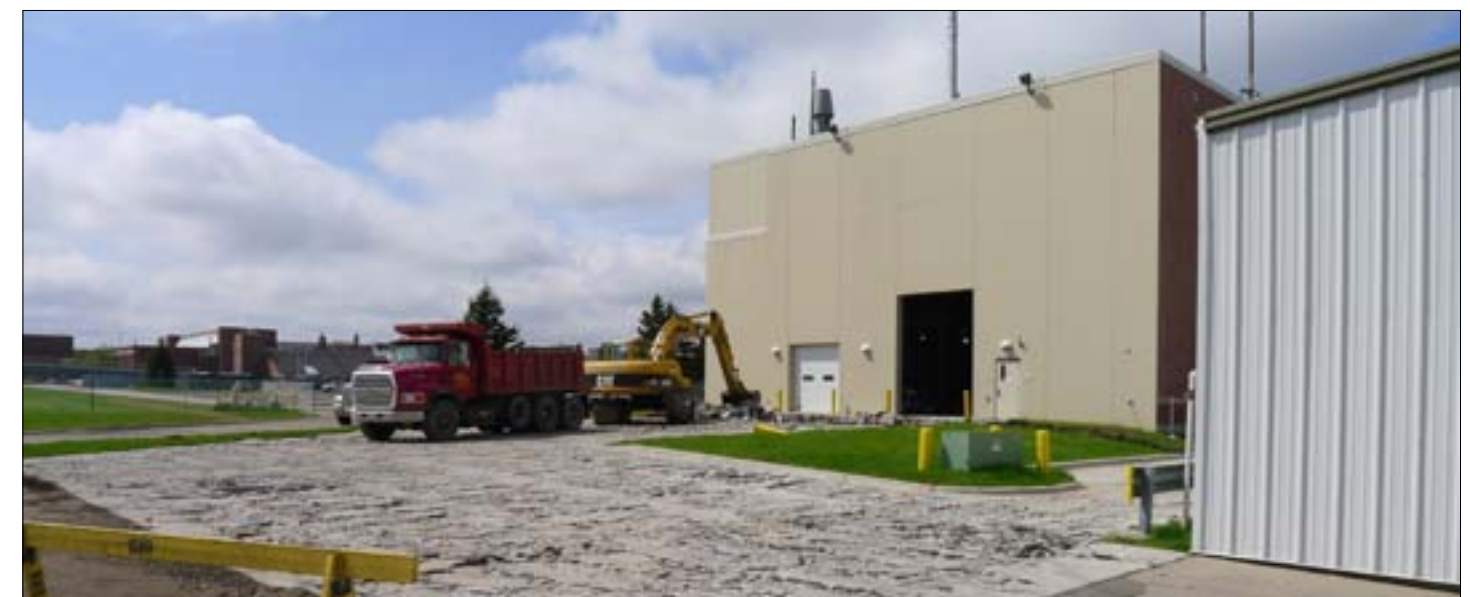
Ground was broken at the National Center for Hydrogen Technology® building in May for an addition that will add a 75-foot (six-level) high-bay demonstration area totaling 18,000 square feet. The addition will house the new Fuels of the Future programs.
