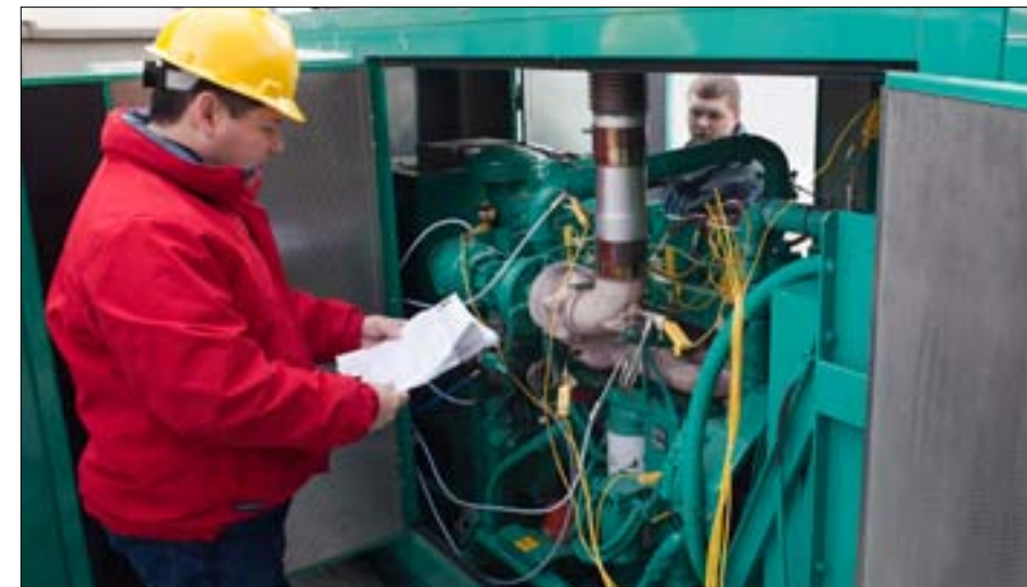
Ismael Chang, Applications Specialist Mechanical for Cummins Energy Solutions Business, assists with the start-up of the syngas-powered engine.
