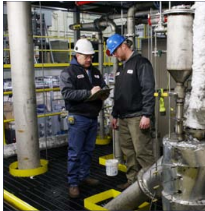
Todd Deibert (left), Technology Development Operator, and Erik Moe, Research Engineer, work on the AFBG, which produces the syngas used in the Cummins generator (see next article).
