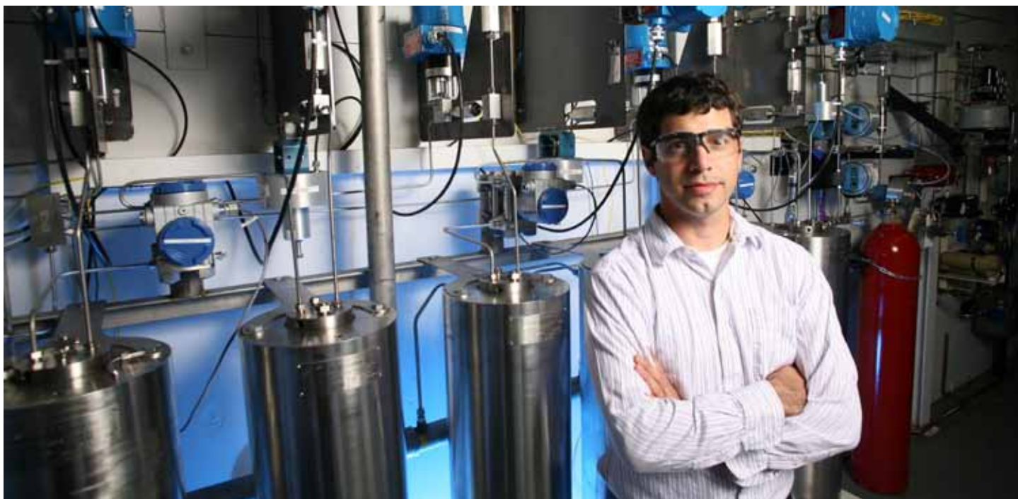
Research Engineer Kyle Palmiscno works with the new pressure swing adsorption equipment used in the hydrogen on-demand process.
